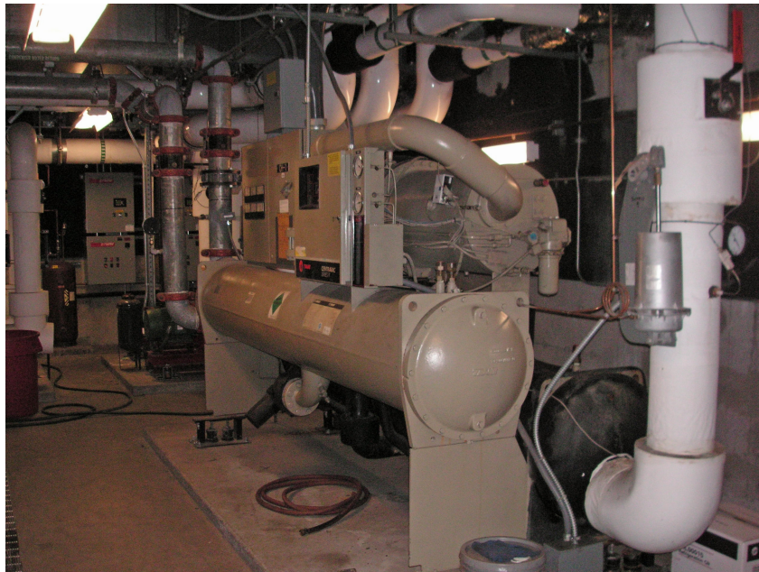
Figure 4: Machine room setting.
