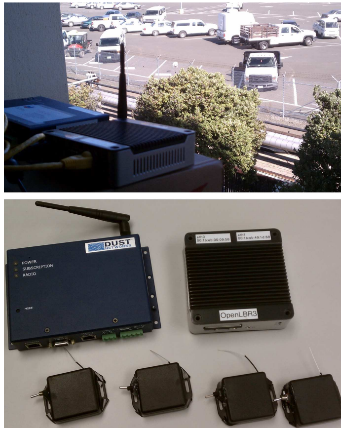
Figure 2.9: Long-term deployment setup at the Chevron-Richmond refinery. The result of this test was a detection rate of 100% with no false alarms. The sensors withstood strong winds and rainy weather.
