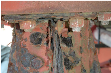
Fig. 14. Rusting on the Bridge
